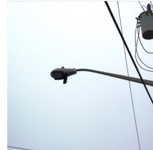
Fig. 2 - Type 1 Street Light located within the parking lot.
